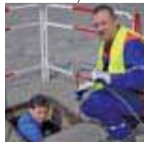
Poland Teamwork at a cable well makes process faster for pulling a new fiber cable.
