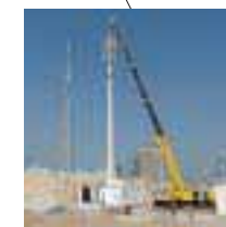
Export Erection of a monopole for GSM network in United Arab Emirates.
