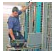
Germany A highly competent field engineer is measuring the quality of a 3G network's core equipment.
