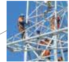
Finland Work safety is a priority for Eltel when working at high levels.
