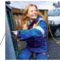
Sweden Broken cable is fixed in Stockholm and power is ON again.
